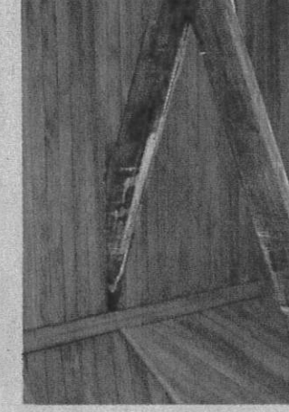
LEAKS: This image shows where water is seeping through the church's sarked ceiling.
